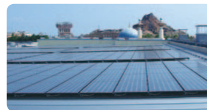
Solar panels installed on the roof of a Company building
