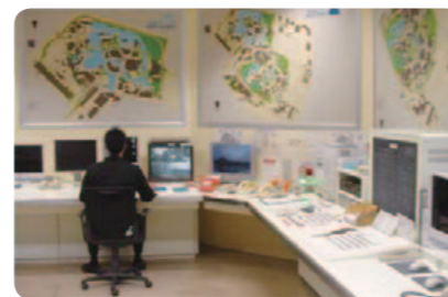
Specialist disaster prevention staff are on duty to monitor the Parks 24 hours a day
