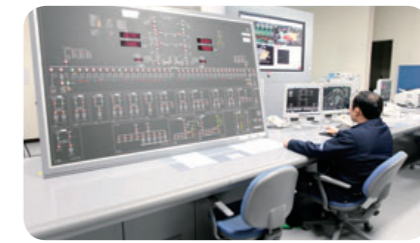
The central energy monitoring system
