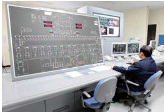
Central energy plant that manages the heat used in air conditioners throughout the theme parks
