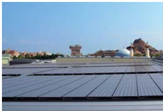
Solar panels installed on the roof of a Company building
