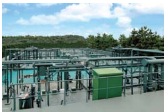
Water is collected and purified at OLC's own water treatment facilities
